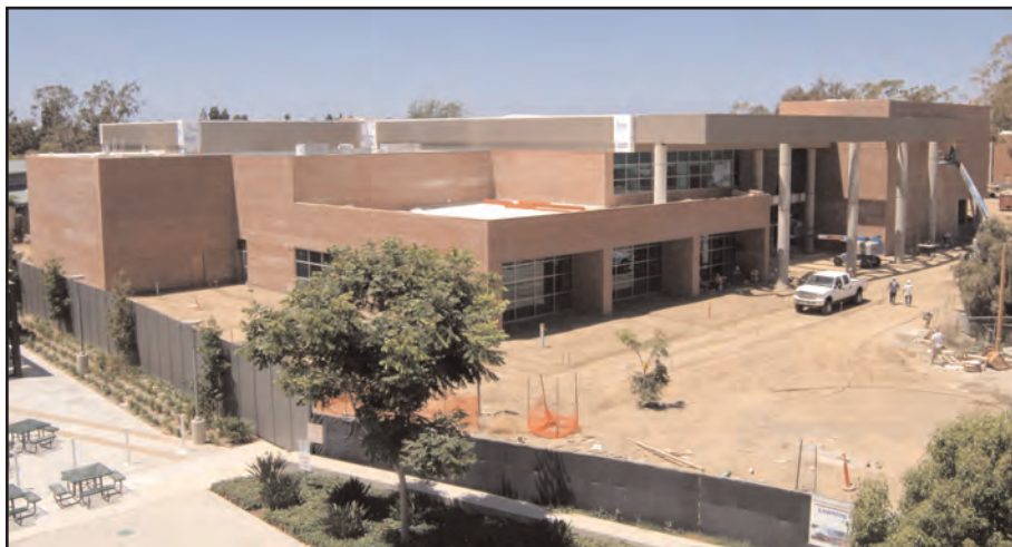
NEARLY COMPLETE - Construction will be finished in December, with a grand opening planned in January 2008.
